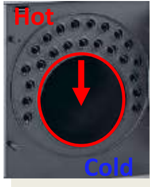
Furnace misalignment against the outer shell
